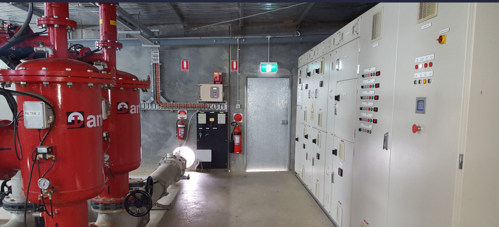
Aldinga Pump Station, Willunga Basin Water Co, SA
